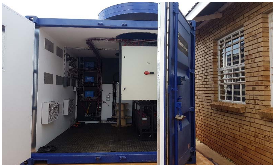
Power Management System including 28.8 kWh Battery Storage
