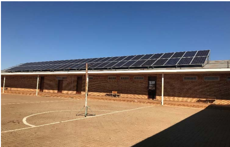
17kW Solar PV System
